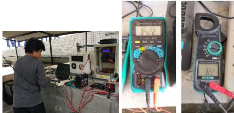
Figure 9. Voltage Measurement of Solar Panels 1 and Solar Panels 2
