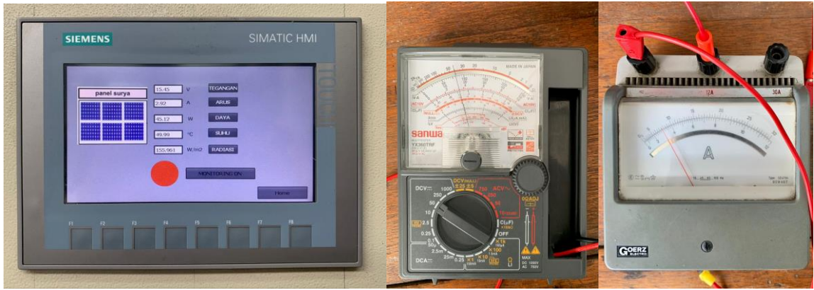
Figure 8. Real time monitoring PLTS
