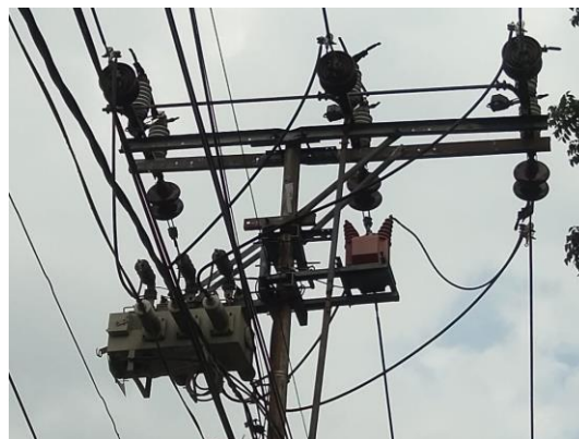
Figure 3. Distribution current transformer installed in the 20 kV distribution feeder
